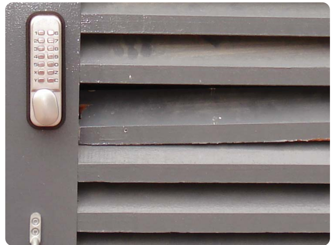
Figure 28: Bad Practice: Thieves gain access by breaking wooden slat to open lock on the inside.
